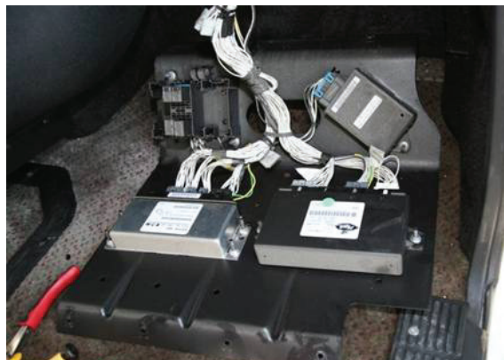
The photo above shows the location of the VECU on a V-MAC III conventional cab truck. The VECU is the module on the right.
